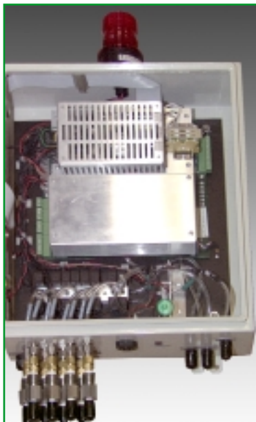
Interior, Chemgard Gas Monitor
